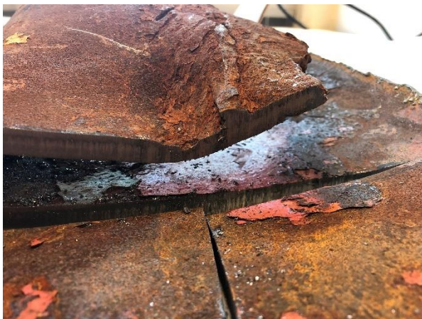
Figure 8 Cross section of the plate in the vicinity of the fracture line (to the right)
