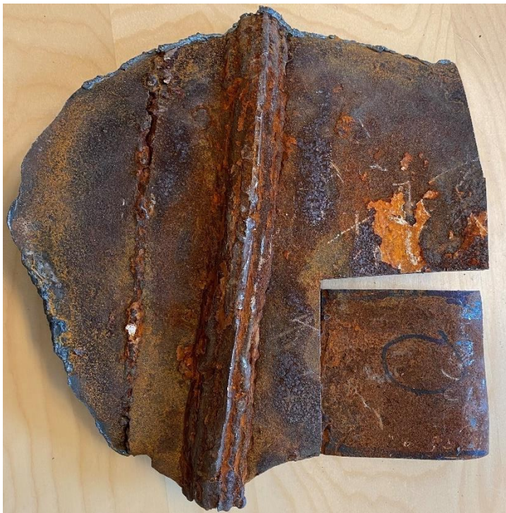
Figure 4 Backside of the plate showing the butt weld and the weld region. Samples are not directly located in the vicinity of any welds.
